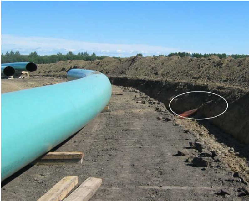
Example of how Excavation may Unearth Wires
