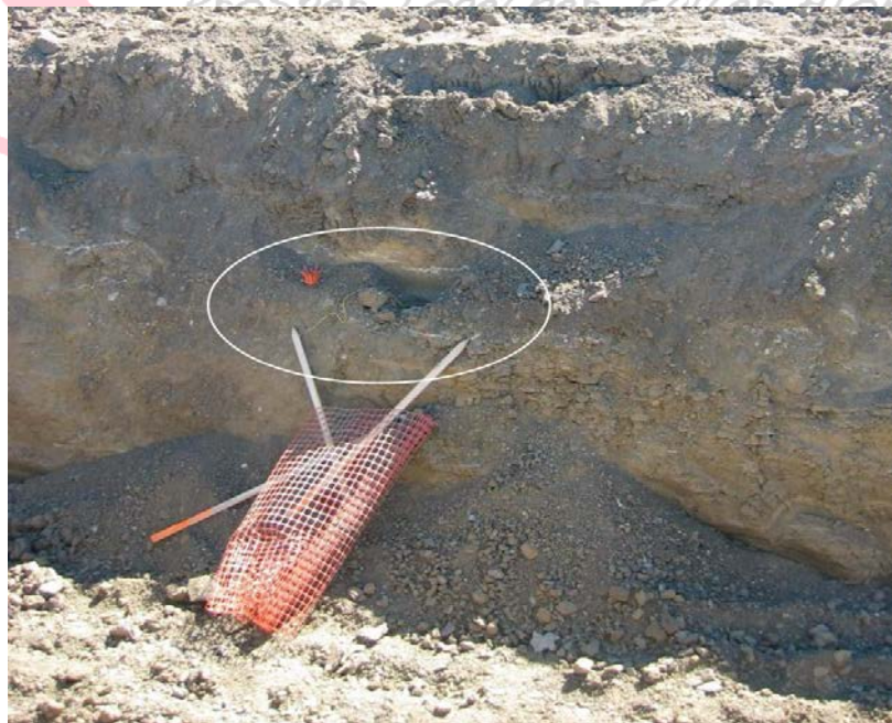
Example of Exposed Wires During Excavation
