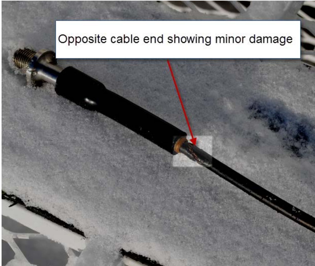
Opposite end of cable showed some minor damage. It is an industry norm to use electrical tape to cover over areas such as these.
