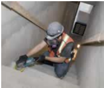
Worker grinding concrete in a stairwell with local exhaust ventilation. Note the exhaust unit at the bottom of the stairs.
