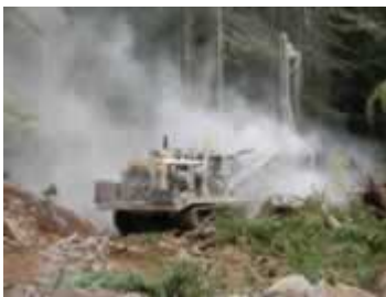
Rock drilling without dust controls.
